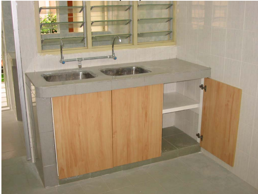
Double sink with concrete tiled worktop in dry kitchen
