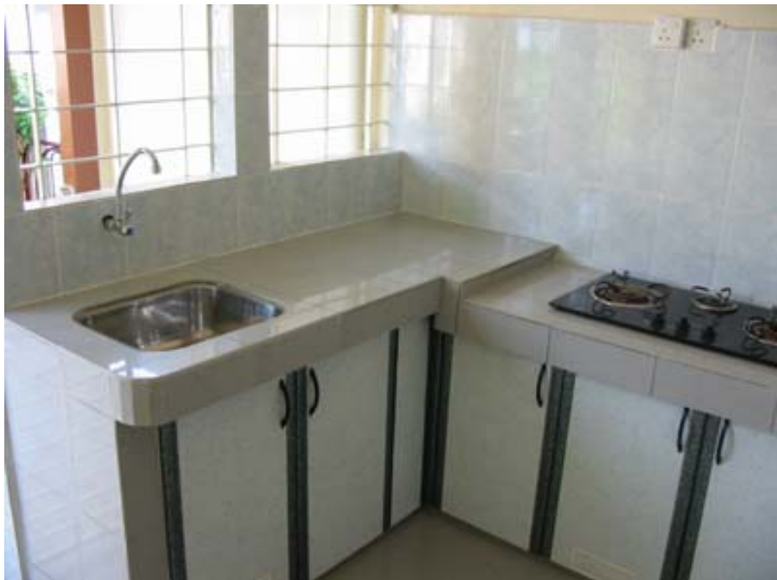
Single sink and extended tiled worktop in wet kitchen with built-in 3-burner stove.
